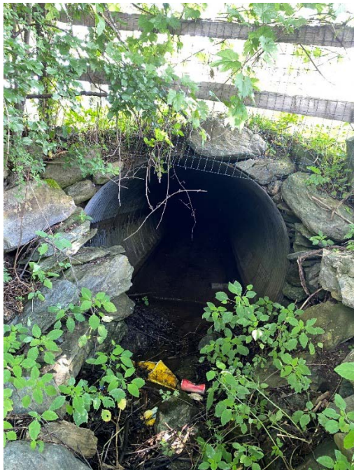
Photo 19. Photograph taken looking generally north at the outlet end of BR 58A where Stream BR58A-S1 flows generally south. Stantec, July 19, 2022
