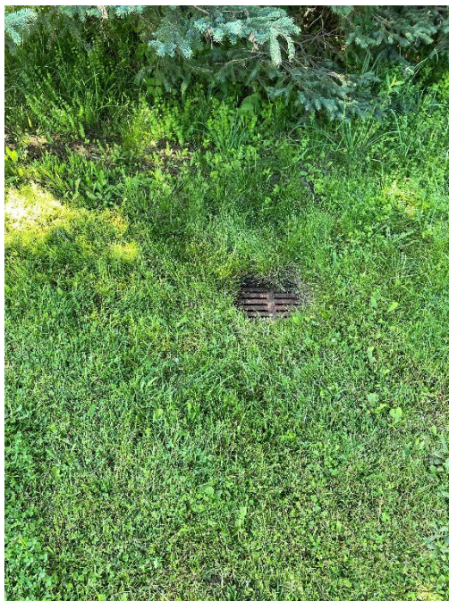
Photo 17. Photo view looking at the inlet of the BR 58A culvert structure in Rupert where it crosses VT-30. Culvert inlet is on the north side of VT-30 within a mowed/maintained lawn area. Stantec, July 19, 2022.
