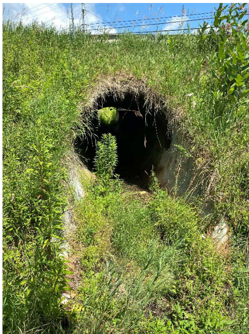
Photo 23. Photo view looking generally north (upgradient) at the outlet end of BR 25 where it crossed VT-11 in Londonderry. Stantec, July 19, 2022.
