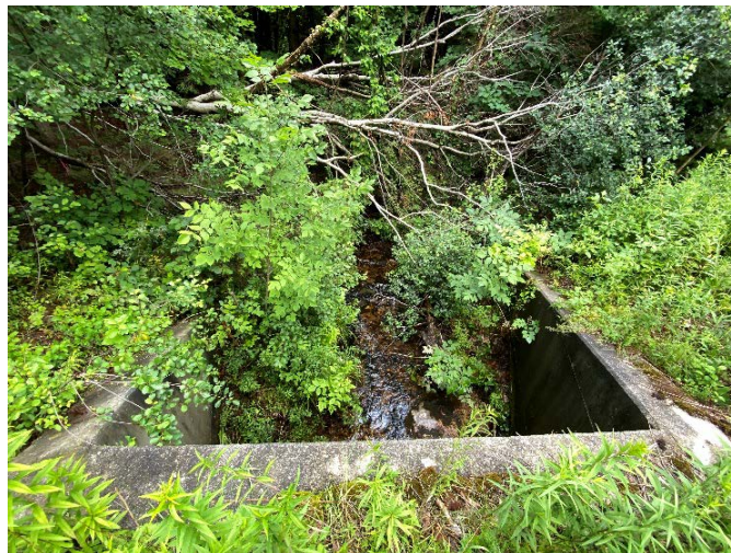
Photo 22. A view looking at the outlet of BR 19-7 on the east side of US-7, photo view looking generally east at vegetative cover downgradient from the crossing culvert. Stantec, July 19, 2022.
