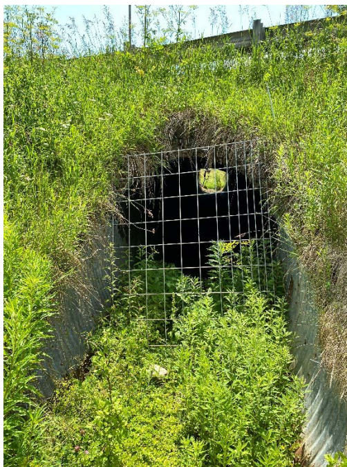
Photo 25. Photo view looking generally south (downgradient) at the inlet end of BR 25 where it crosses under VT-11 in Londonderry. Stantec, July 19, 2022.
