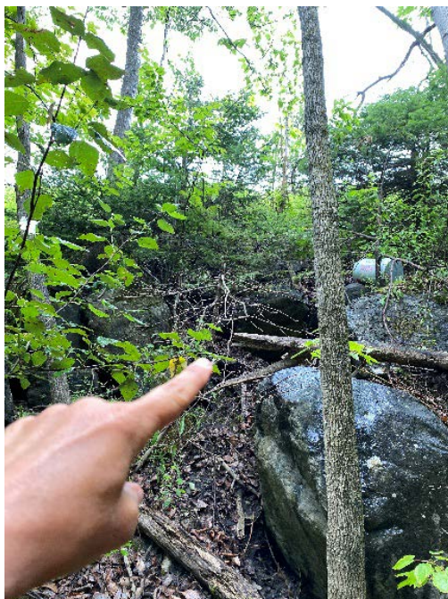
Photo 8. A view looking generally south towards US-4 and the assumed approximate location of the upgradient/inlet end of the BR 28 culvert (culvert not found in field, appears to have been buried by fill, debris, organic material, other). Stantec, July 18, 2022.
