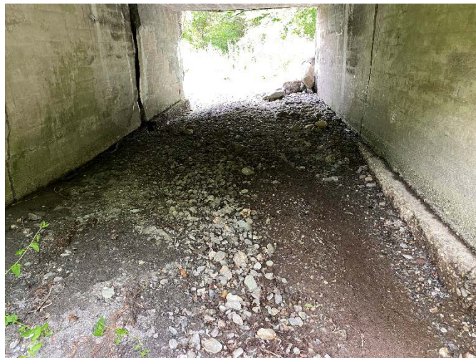
Photo 4. A representative view of conditions in the BR 14 culvert crossing of VT-4A in Ira. Photo view looking generally north. Stantec, July 18, 2022.
