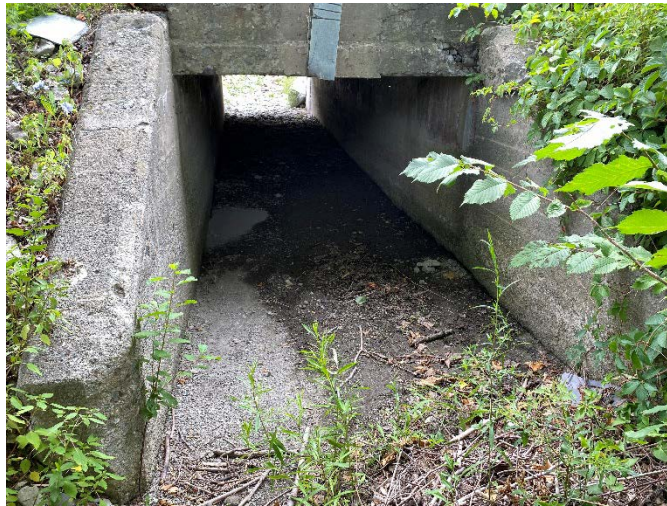
Photo 1. View looking south through the BR 9 culvert under VT-4A in Castleton. Stantec, July 18, 2022
