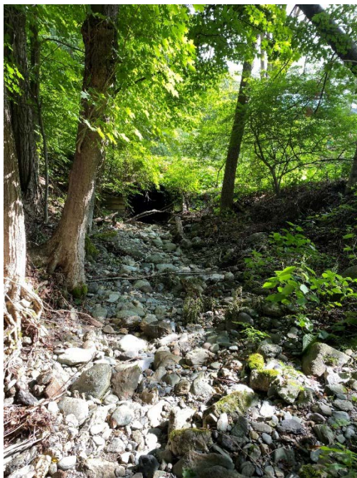
Photo 15. Photo view looking north towards the inlet of BR 61 where it crosses VT-30. Photo view shows culvert dry streambed conditions and some evidence of dynamic channel with exposed roots on mature trees. Stantec, July 19, 2022.
