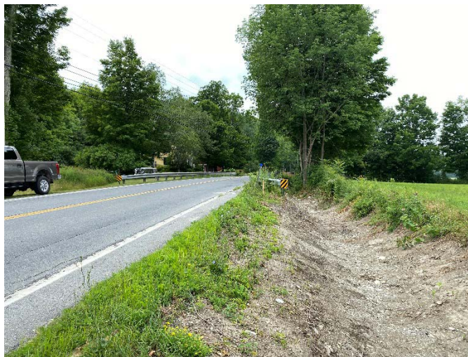
Photo 2. A representative view of recent ditch excavation work on the north side of VT-4A, downgradient from the BR 9 culvert crossing. Photo view looking generally west. Stantec, July 18, 2022.
